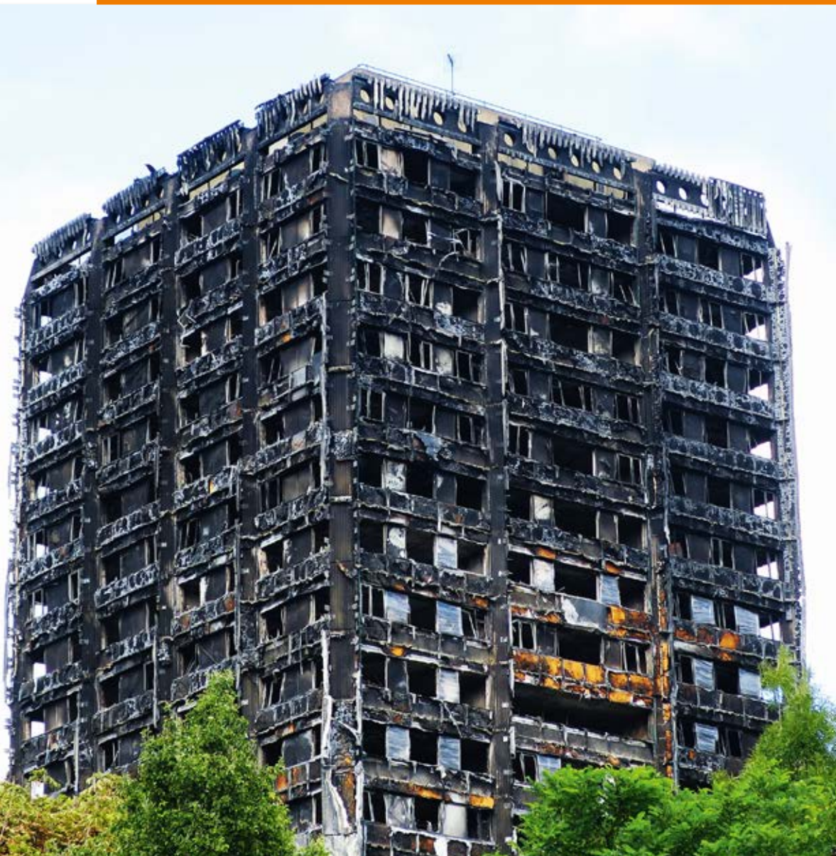
79 people died when a fire broke out in the Grenfell Tower in London. A pressure differential system could have saved those lives.
